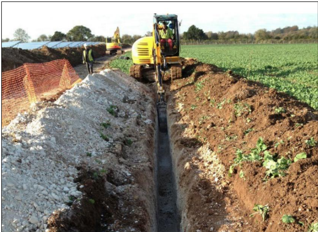
Plate 3: Cable trenching, showing topsoil stripped and set to one side, with subsoil placed on the other side ready for reinstatement (image courtesy of British Solar Renewables)
